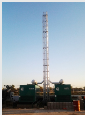
DG EXHAUST PIPE & CHIMNEY
