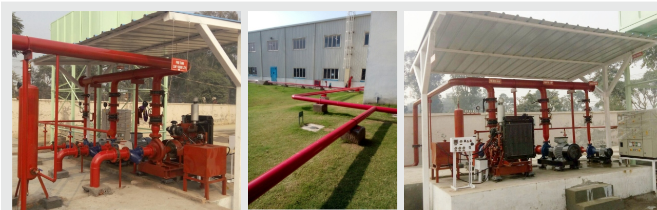
PROJECTS FIRE FIGHTING SYSTEM
